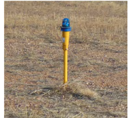
Medium Intensity Taxiway Edge Light (MITL)
